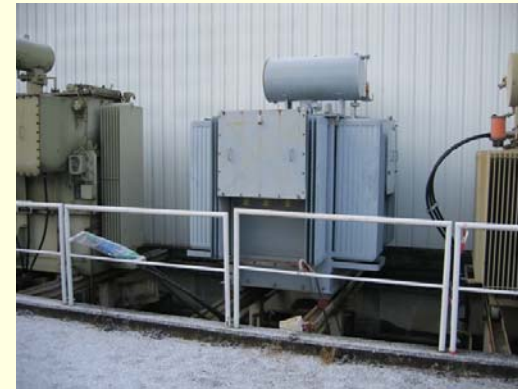
AC transfo outside build.193
