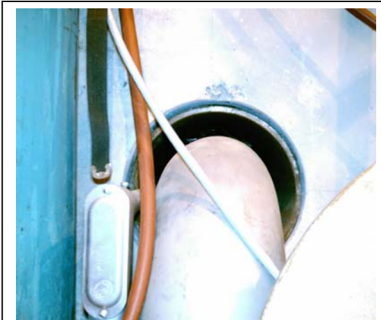
Annular space around water line proposed for use with the gaseous N2 vent.
